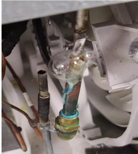
Technician connection leaking
