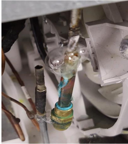
Technician connection leaking
